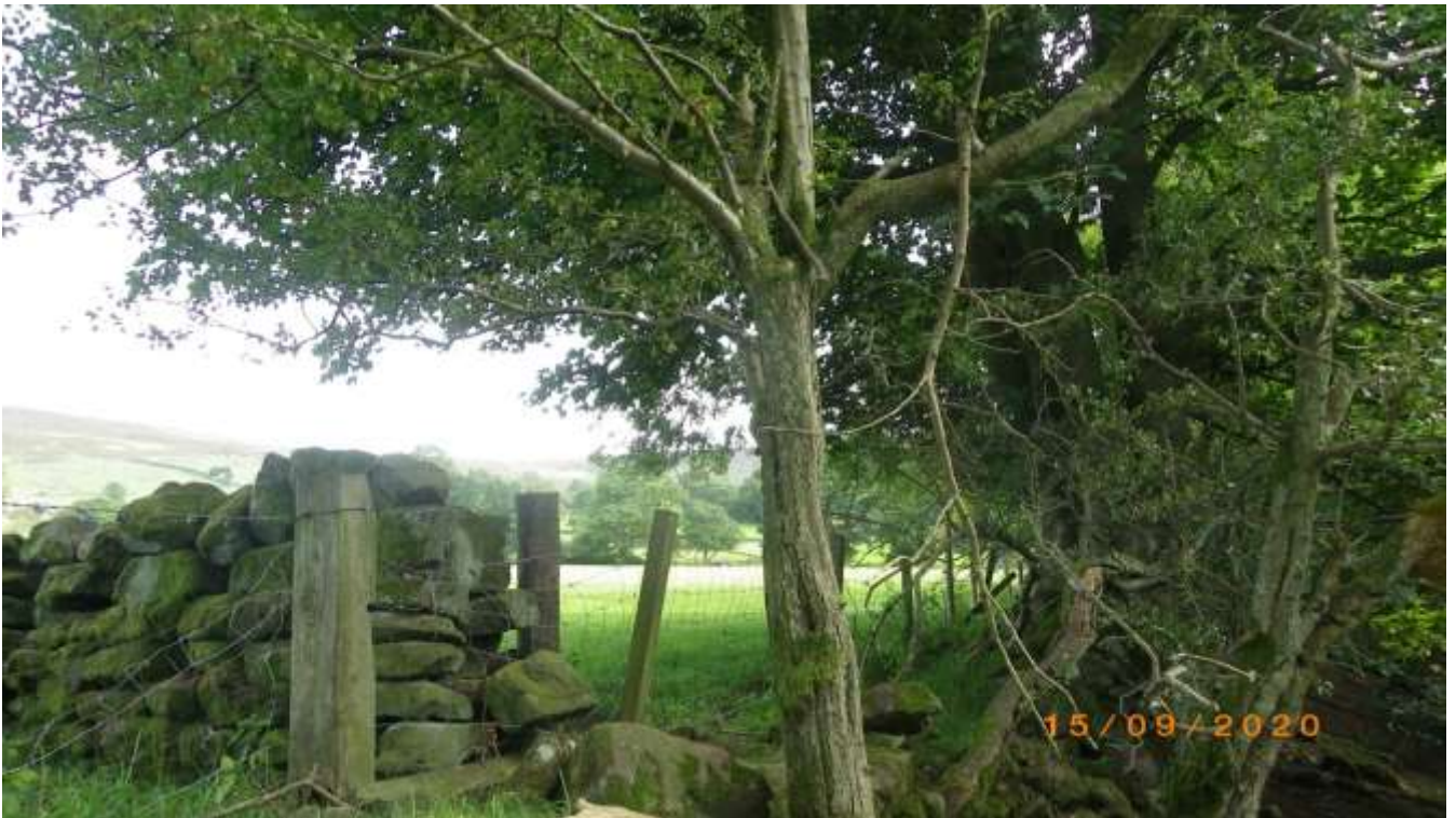
Photo 142 cpy9a eastern boundary poor condition in parts
