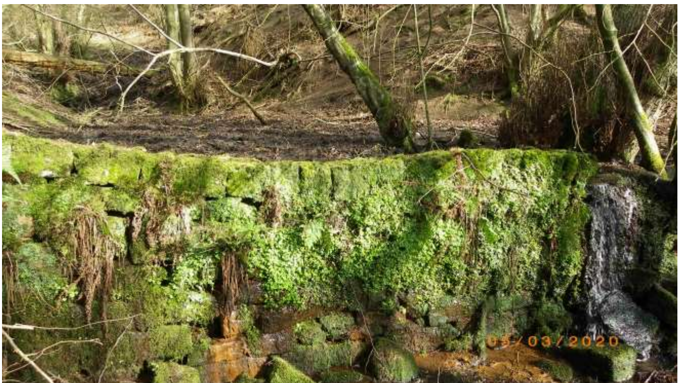
Photo 460 Cpt28 Hall Wood watercourse going over the top rather than using culvert
