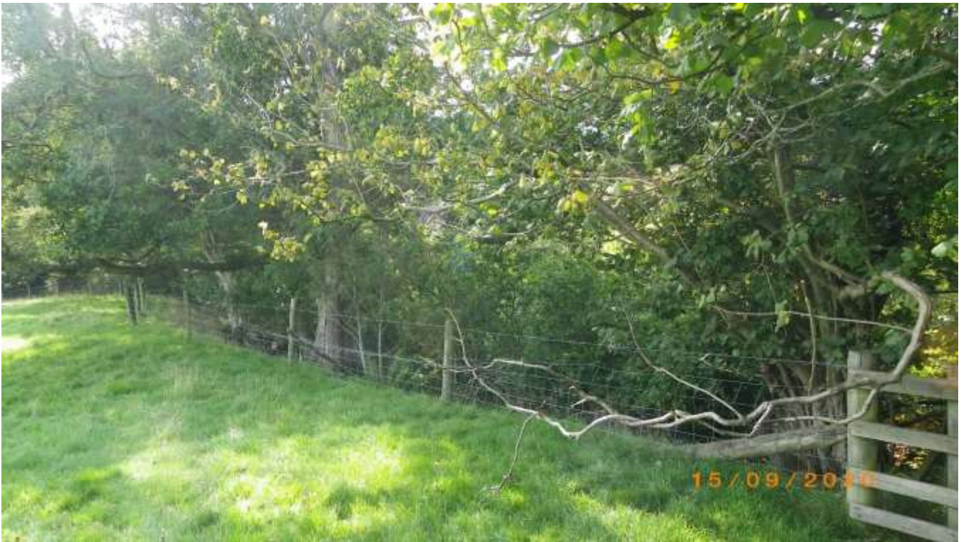
Photo 164 Cpt10b some fences in poor condition; see brown thick line on map 14
