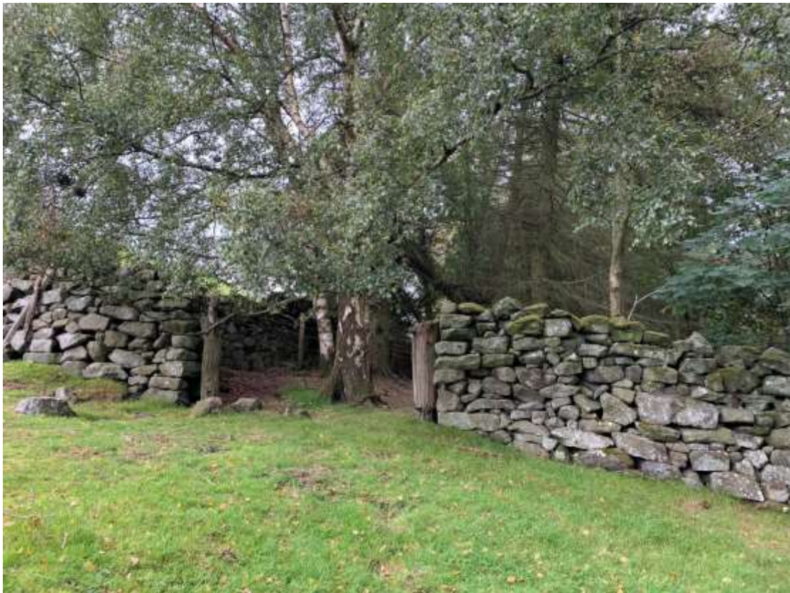
Photo 425 Cpt24a Shawbeck Wood boundary wall on east of wood not stock proof
