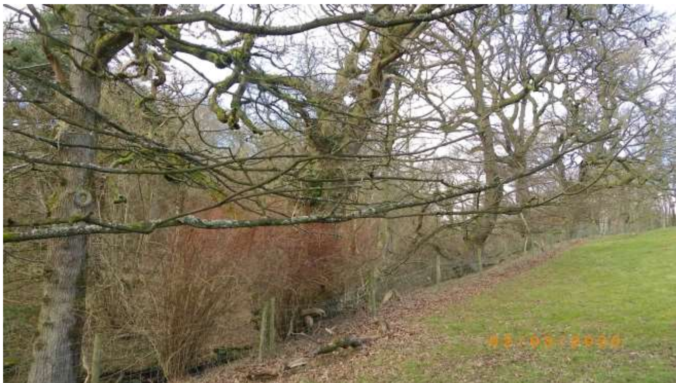
Photo 15 South east boundary of 1c stock fence to grass field is old.
