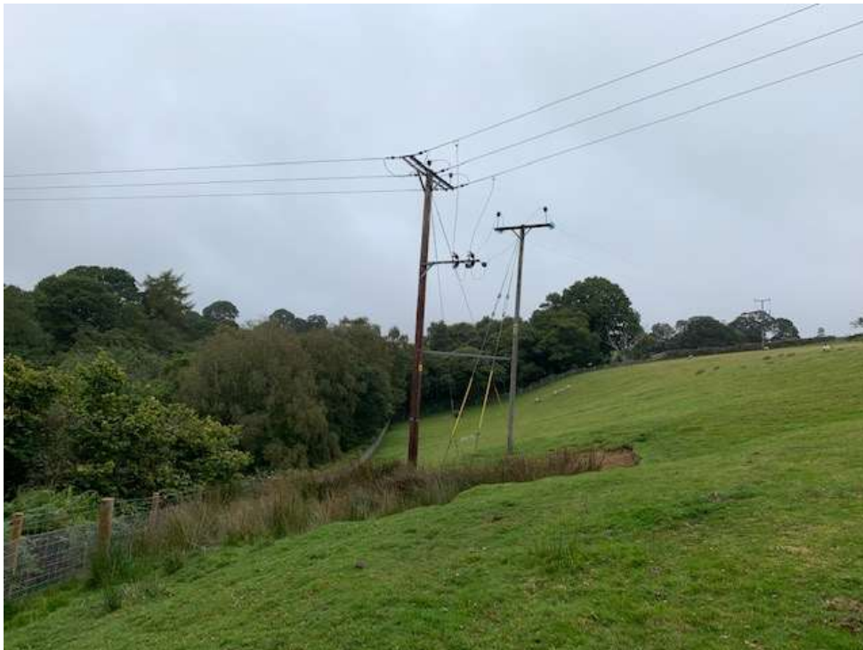
Photo 405 Cpt22a Overhead electric crossing Low Wood
