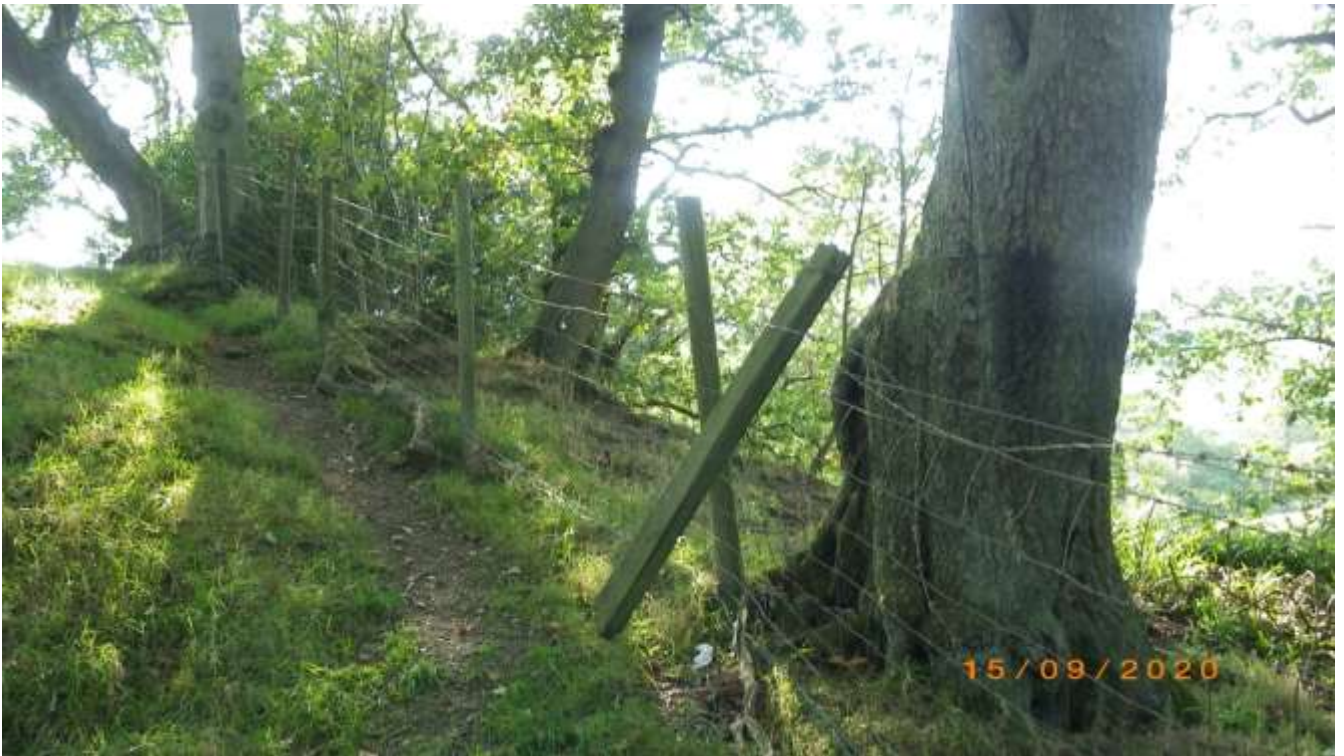
Photo 170 & 171 Cpt10a poor fence condition to south of wood
